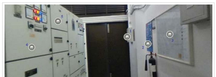
Figure 2: Screenshot of VR Training view within switch-room.
